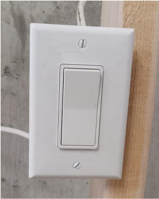
Figure 10. Secure the light switch and cover plate
