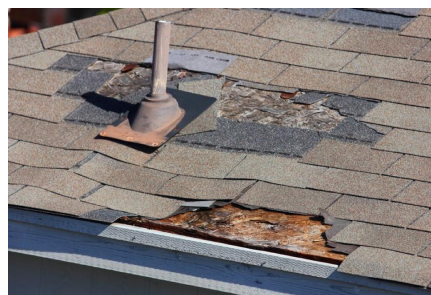
Figure 2. Damaged Shingles and Rotted Roof Deck. (Source: mullinsgc.com)
