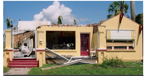
FIGURE 1. Failure of Roof Structure Due to Window Failure During Hurricane.
